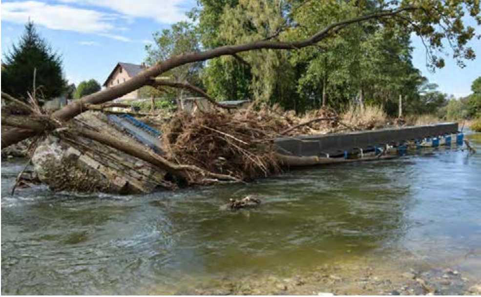
Examples of damage to pedestrian bridges: span displacement from supports – the bridge deck lies in the river. Right photo: uncontrolled settlement of a pier due to scouring of the riverbed.
