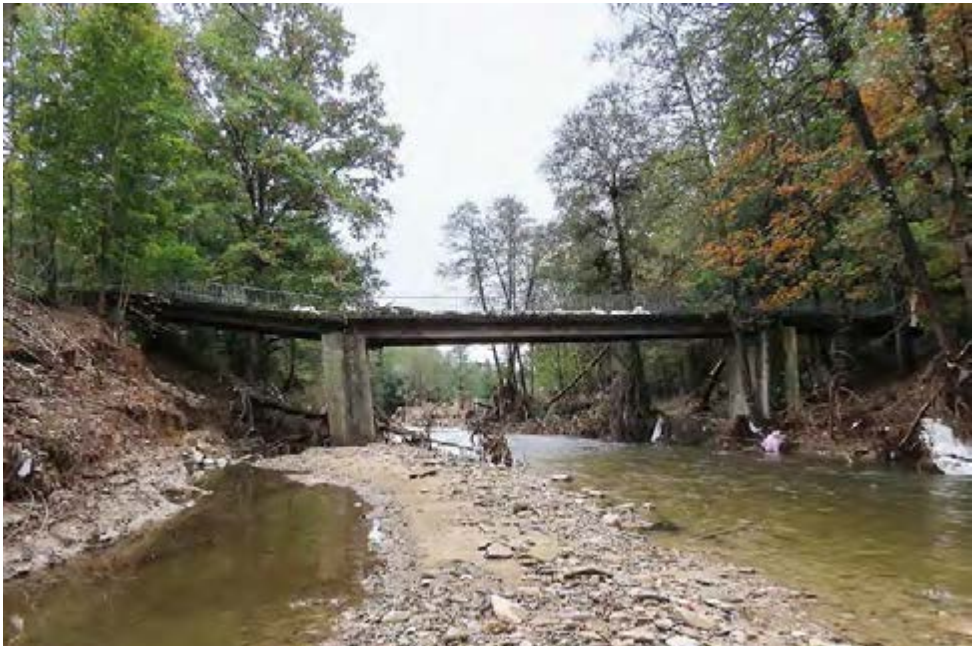
Examples of damage to pedestrian bridges: uncontrolled settlement of a pier due to scouring of the riverbed.
